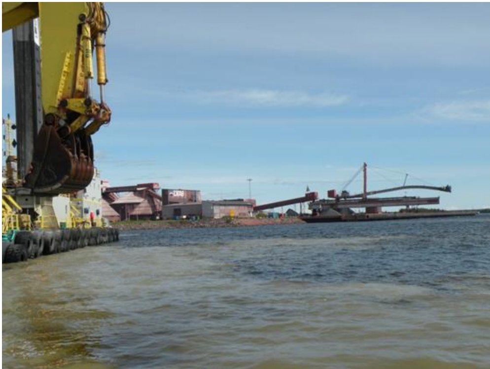
Figure 8: High TSS concentrations (+100 mg/l) were often observed in the vicinity of the excavation observations.
