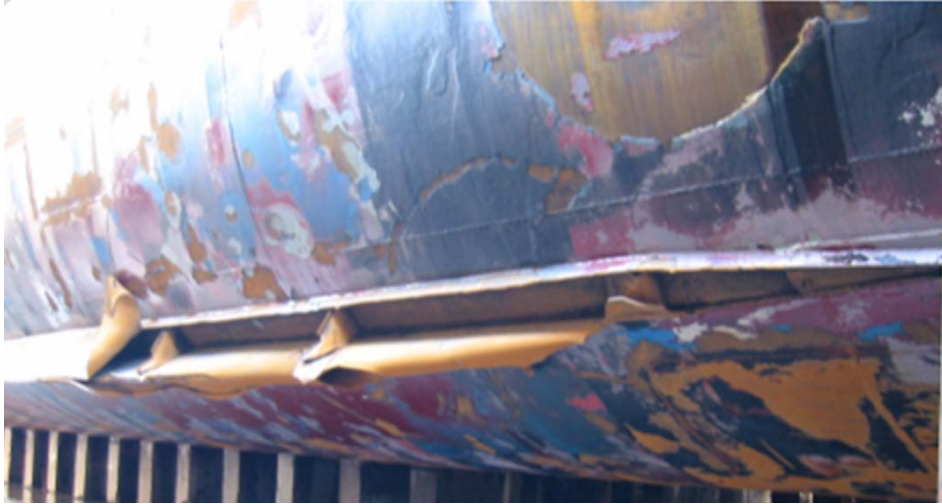
Figure 11. Damage caused by ice on the bilge keel of a ship. Note that this is an example of damage caused by ice, not an example of a good or bad design.
